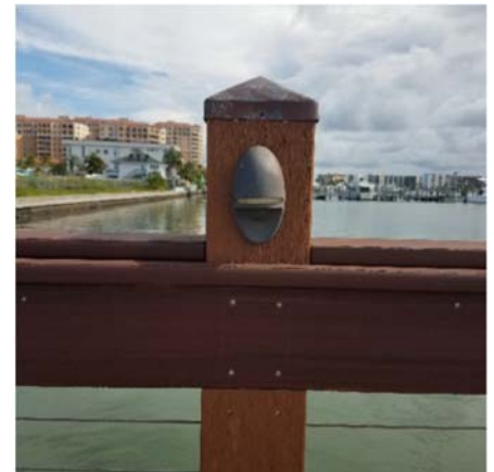
AZEK Accent LED post-mounted light fixture provided by the developer.
