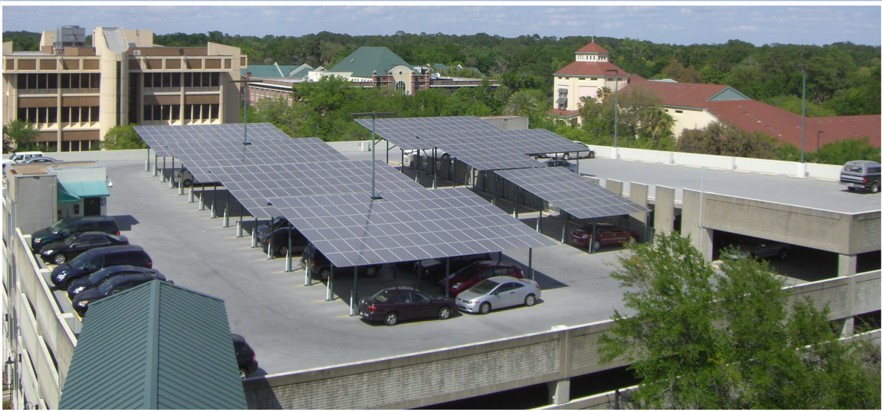
Solar photovoltaics harvest energy while shading vehicles atop the Downtown Parking Garage. (Source: Solar Impact, Inc. and McGurn Management Company)
