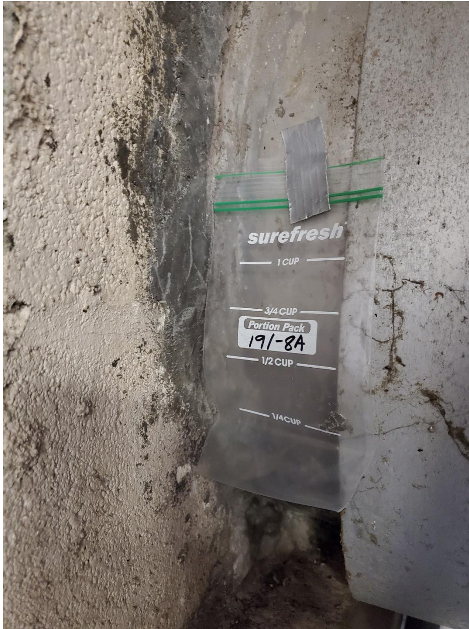
191-8A: Generator Exhaust Patch [NAD]
