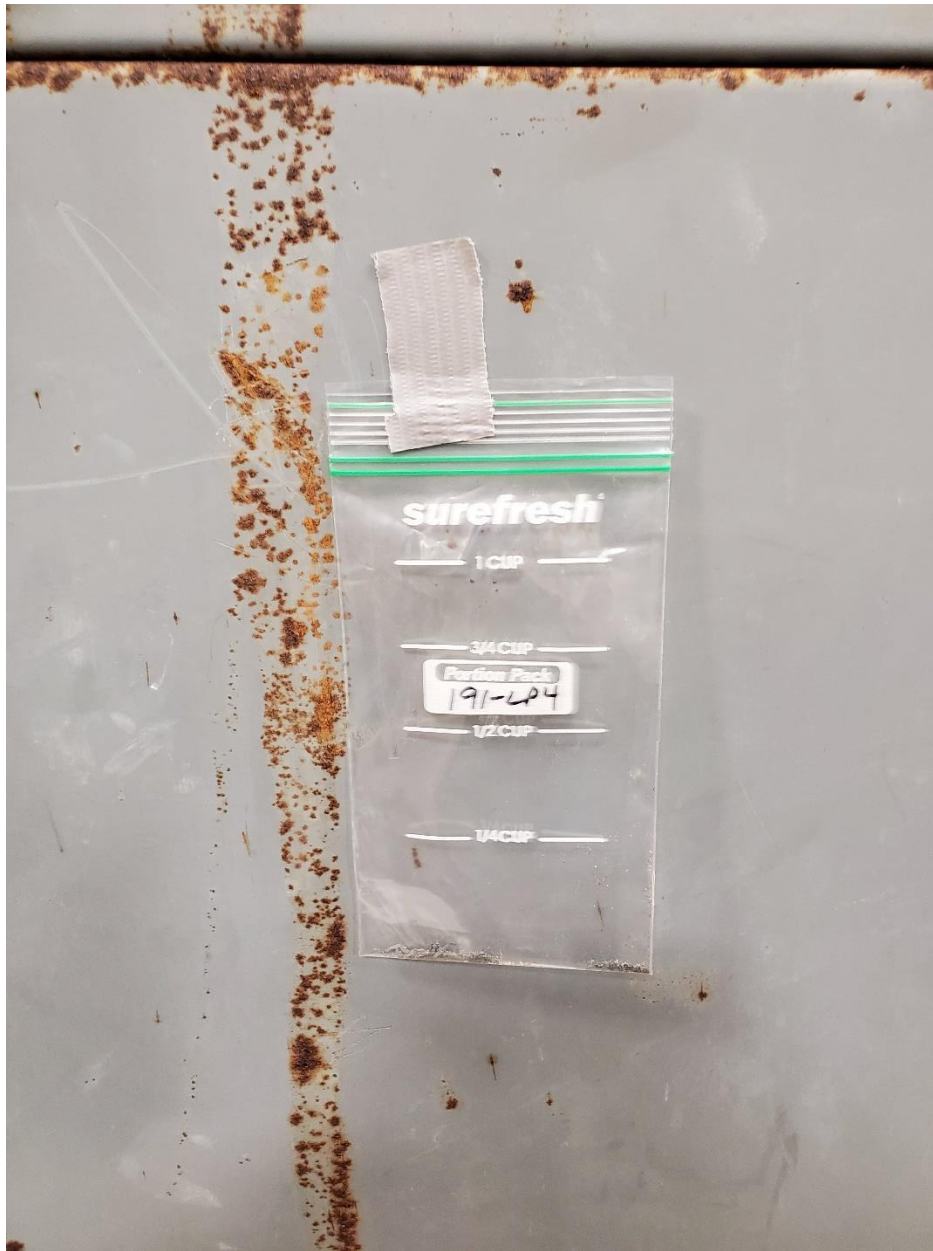
191-LP4: Dark Grey Paint on Electrical Components [NLD]
