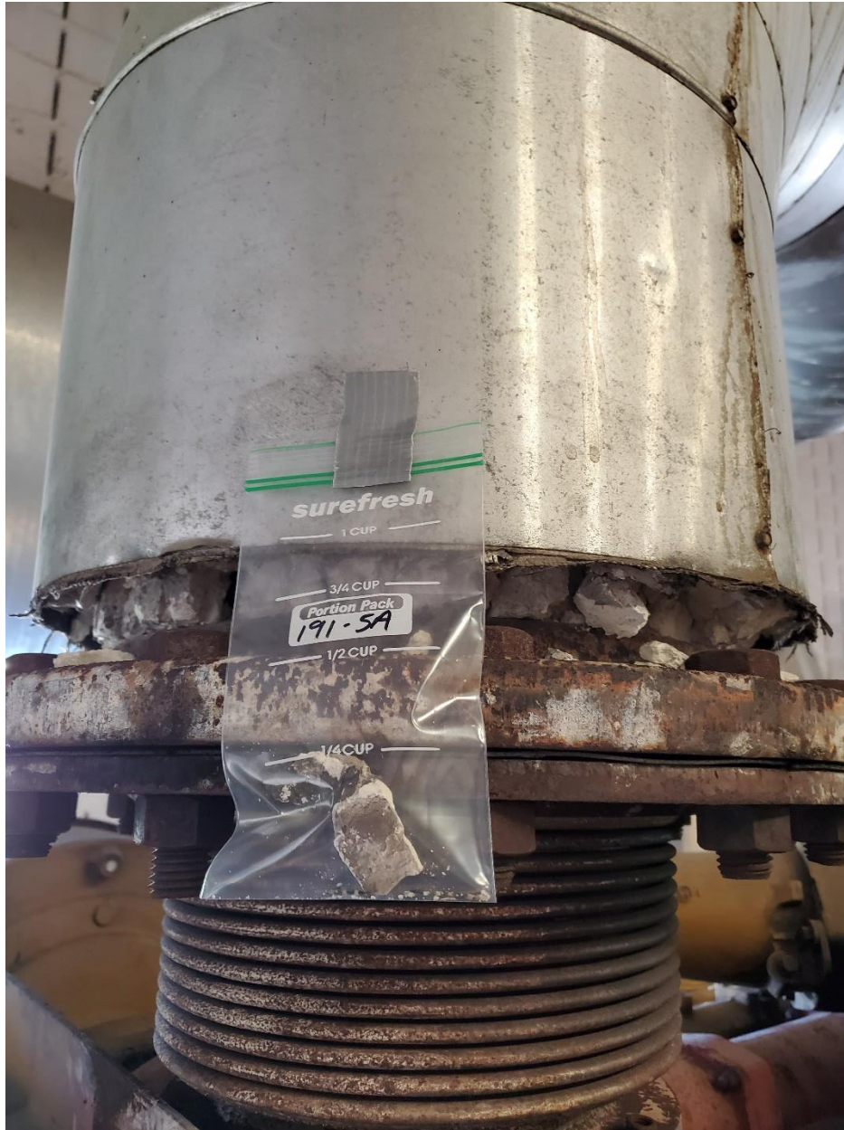
191-5A: Generator Exhaust Insulation [NAD]
