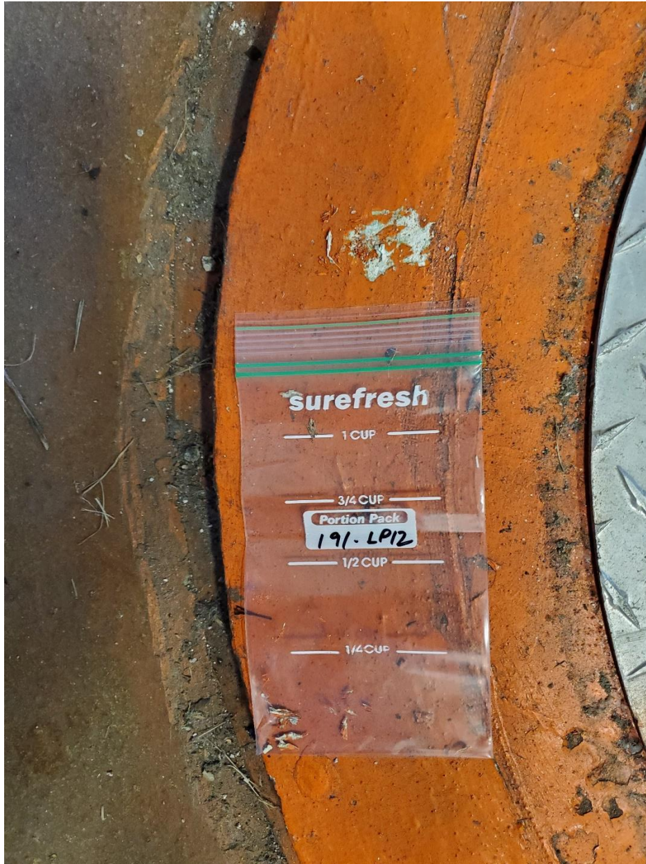
191-LP12: Orange Manhole Paint [NLD]
